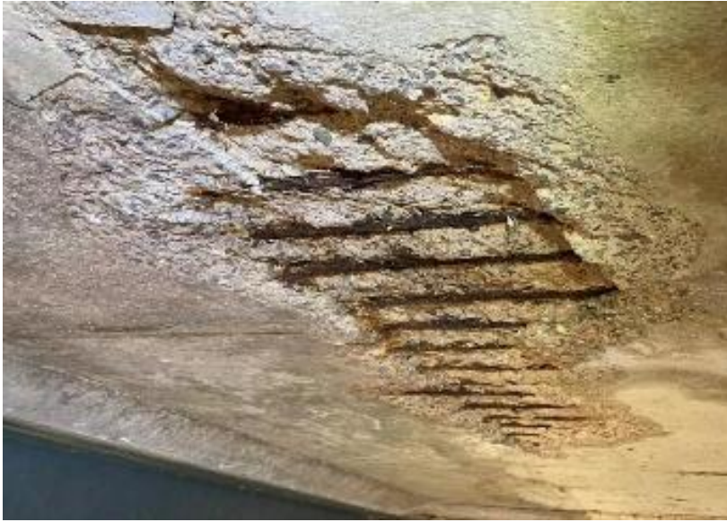
Spalling underneath the bridge
