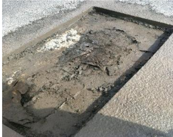
Waterproofing failure and damage to deck concrete.
